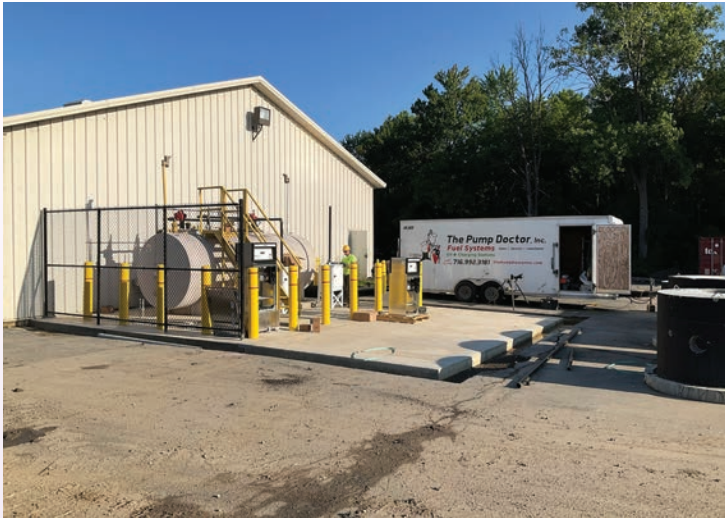
New fuel pad complete and relocation of existing fuel tank in progress
