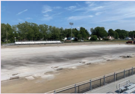
Regrading of the subbase at Howe Field with new choker course stone in preparation for the shockpad and new turf
