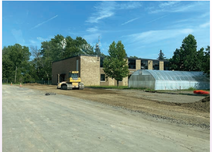
New sidewalk and parking lot resurfacing preparation at the north parking lot
